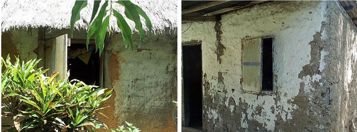
Figure I.1. Typical examples of Melanesian house in New Caledonia, where the wooden structure is covered (internally and externally) by walls of raw earth and tremolite-Pö whitewash. Strong alteration and leaching are visible on the parts exposed to weather (Quénel and Cochet 2001).
